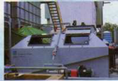
Induced Air Flotation Unit (IAF)
